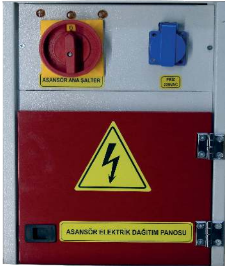
ELEKTRİK PANOSU ELECTRIC PANEL
